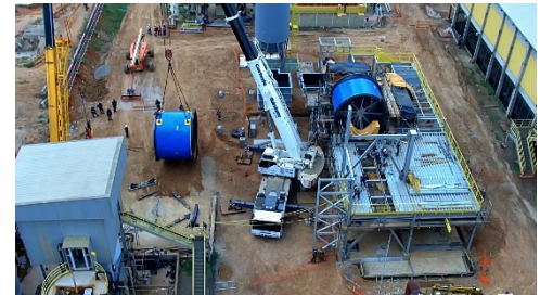
Secondary grinding – ball mill installation
